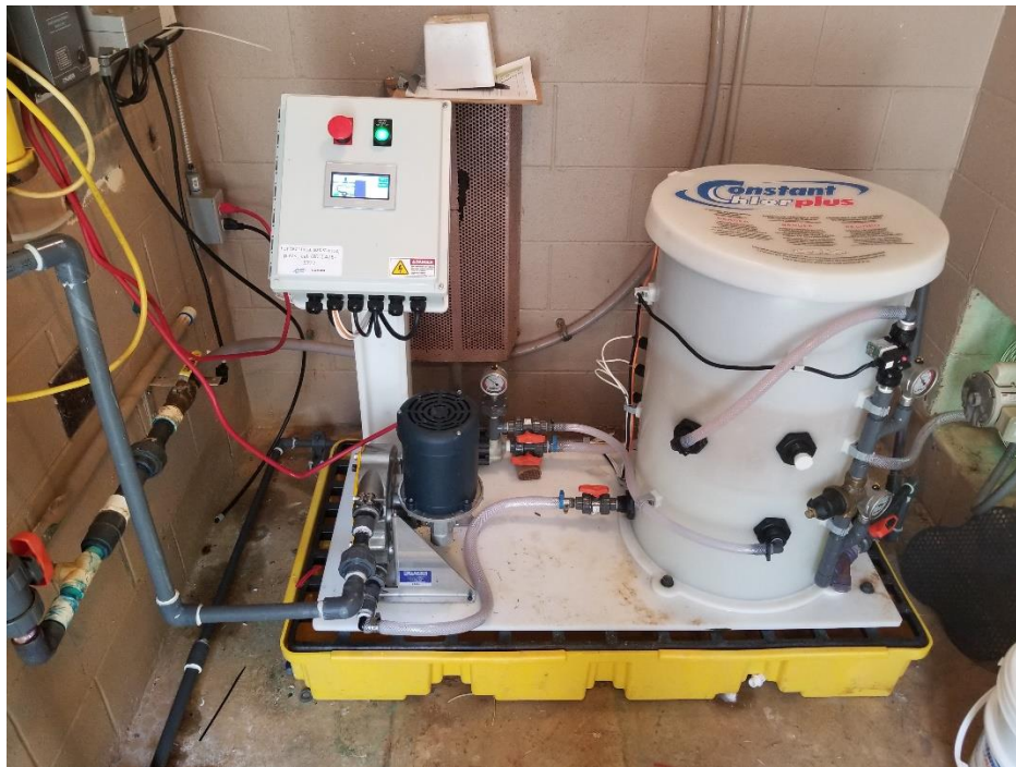
50 PPD Constant Chlor System at Hamilton Co Waste Water Plant
