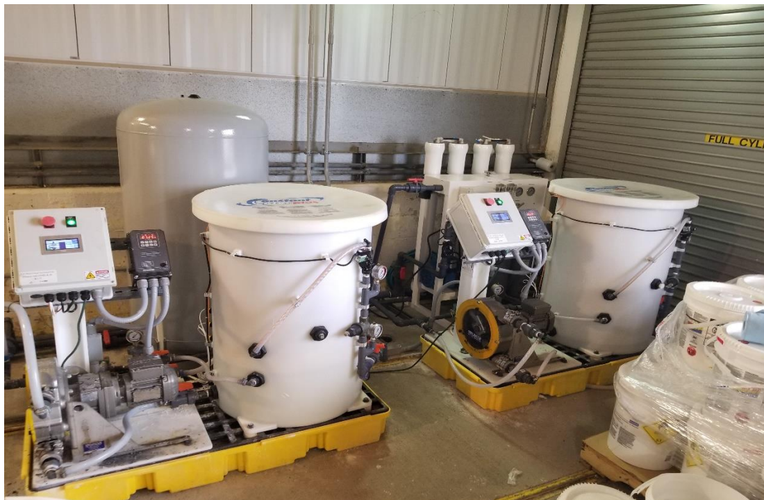
Duplex 150 PPD Constant Chlor Systems at a TN Water Treatment Plant.
